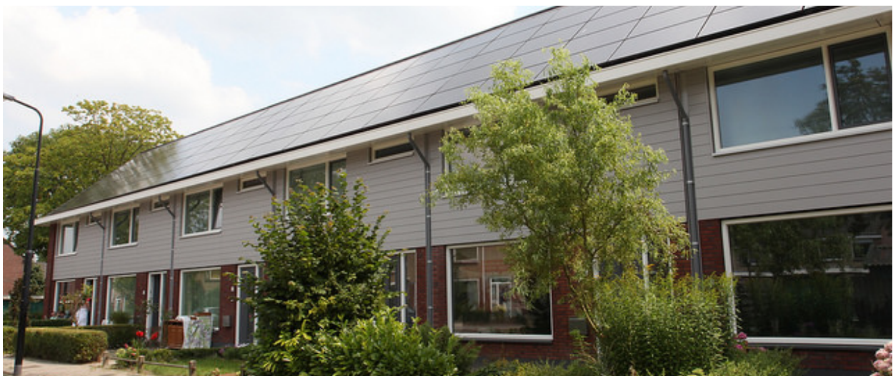
Set of E=0 refurbished row houses, each house is individually measured and it's package custom made
